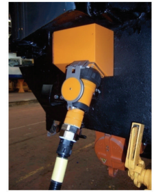
VN-PC Jumper Cable Assembly on Outside of Car
